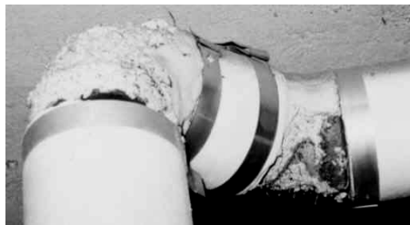
Damaged Pipe Insulation
